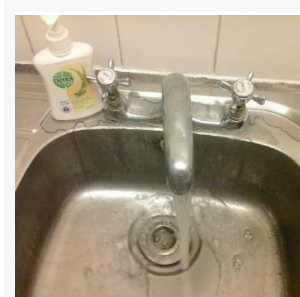
tap is leaking 29/11/2016 10:28 (GMT)
